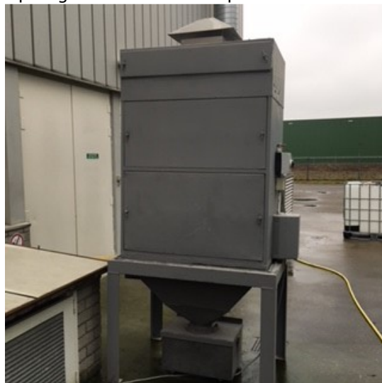
Stofferfilter (dustcheck), lamellen, unit 2
